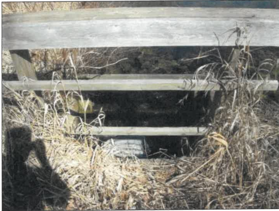
Above: Vertical standpipe allowing flow to pass under road crossing dividing Wetland A and Wetland AA
